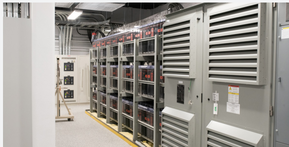
66 TH STREET WAREHOUSE TIER III DATA CENTER
