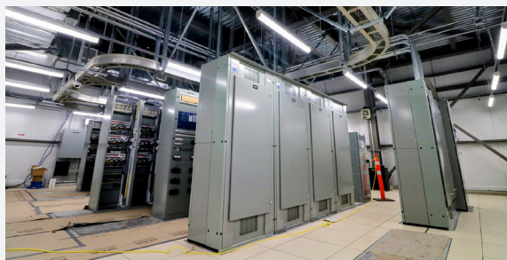
MAINWARING SUBSTATION UPGRADE
