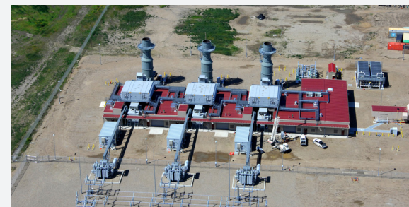
YELLOWHEAD POWER STATION
