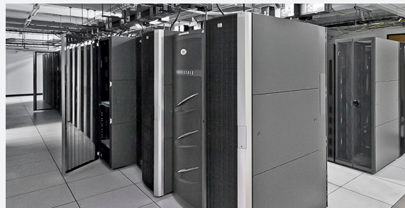
USPS DATA CENTER
