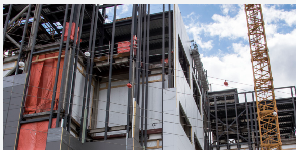
GILEAD - PROCESS TOWER
